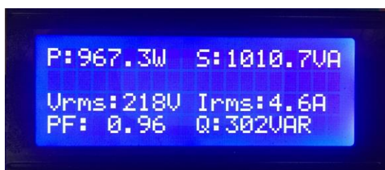
Fig.17: Condition of Load after APFC
